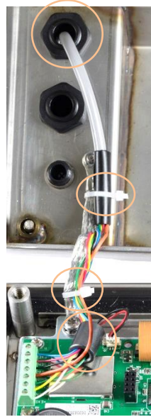
Figure A-24: Analog Load Cell Pin Grounding and Ferrite Installation, IND236
