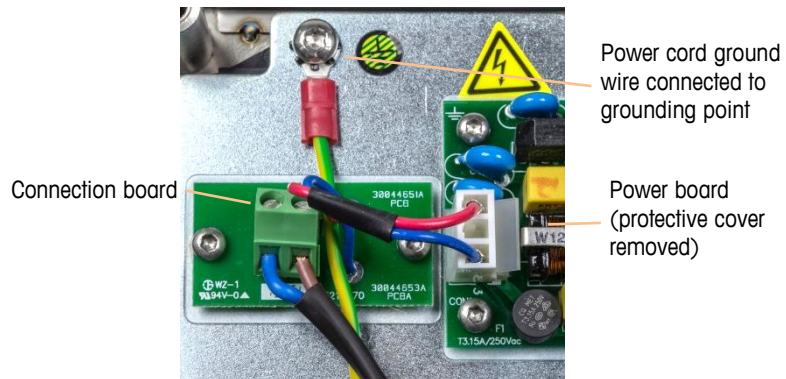
Figure A-18: IND236 AC Power Connection Board and Grounding
